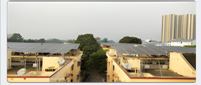
Metro Railway 360 KW – Kolkata, West Bengal
