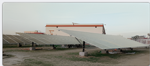
HPCL 120 KW - Kanpur, Uttar Pradesh
