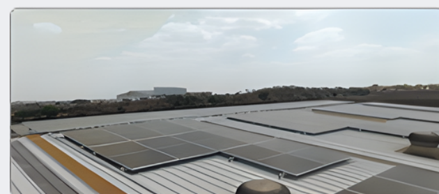
Real Foundry 95.04 KW - Rajkot, Gujarat
