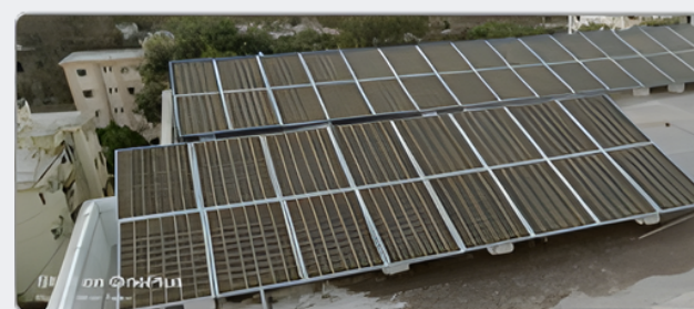
CPWD Branch Office 85 KW - Surat, Gujarat
