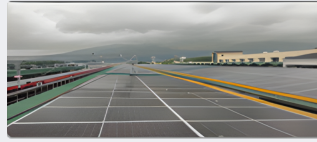
Moradabad Division Railway 479 KW – Moradabad, Uttar Pradesh
